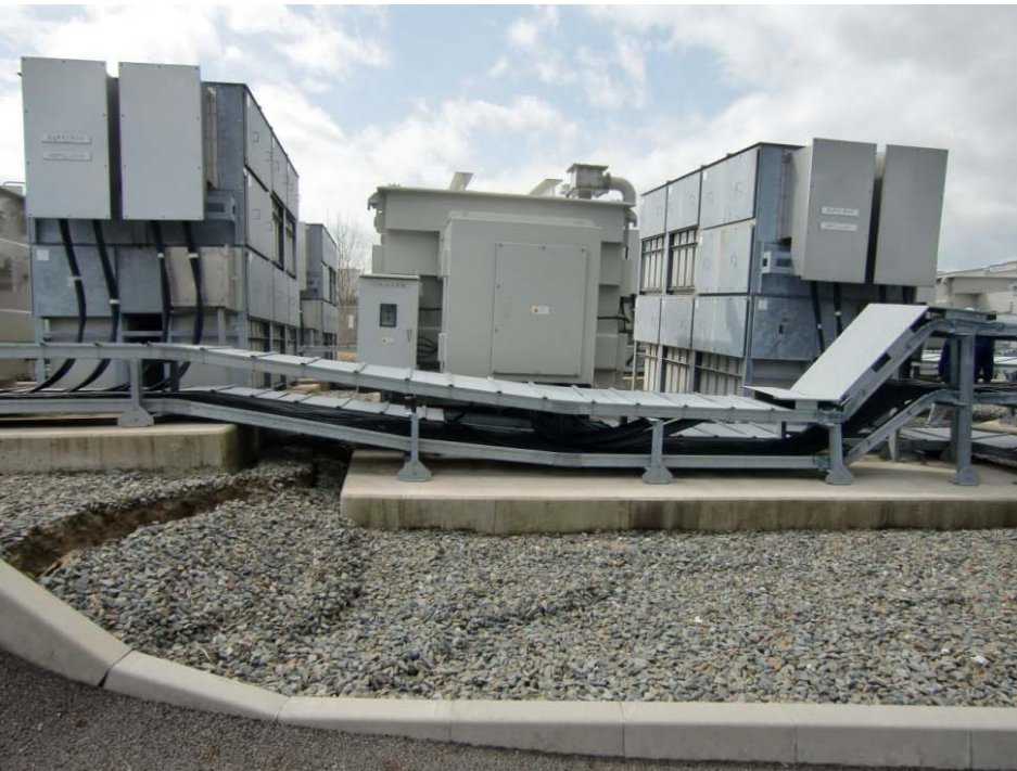
Condenser Bank for 3 GeV
